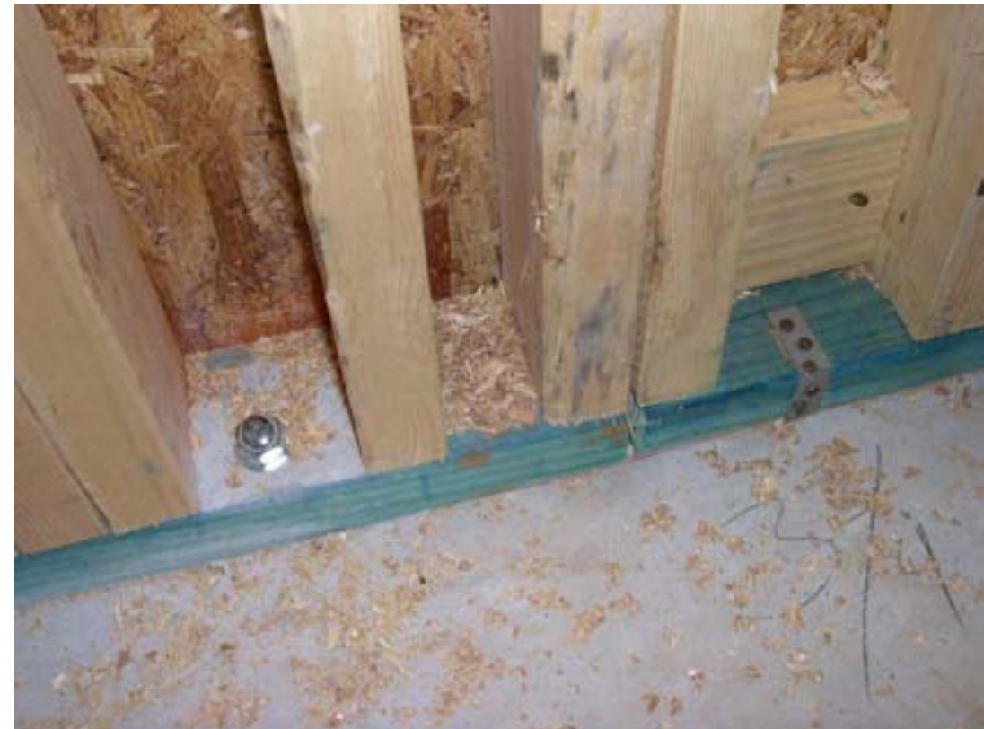
Panels set on bottom plates, anchored with bolts and straps in Georgia
