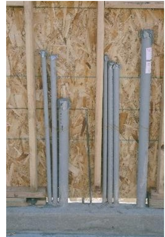
Utilities stubbed into an open-wall panel system
