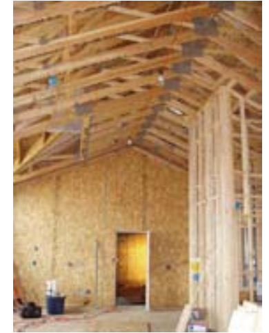
Wood SIP house under construction in Colorado, with infill partitions and wood-truss roof
