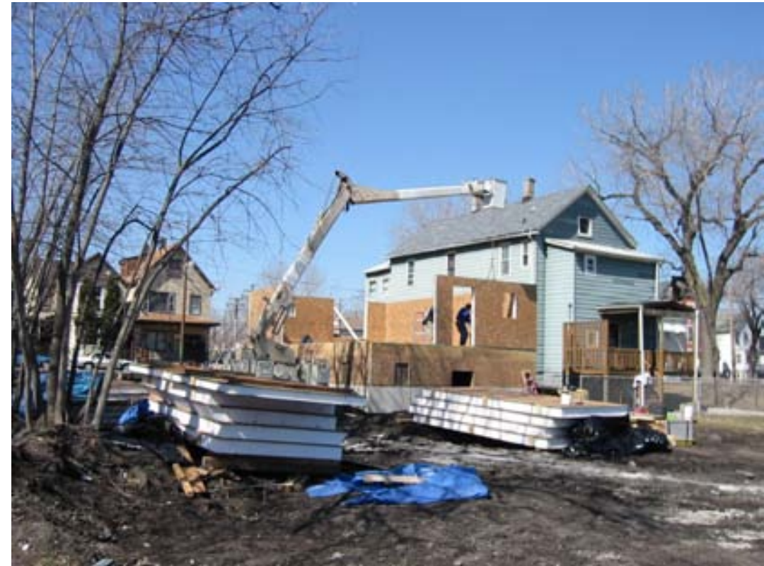
Structural insulated panels are set in place with the aid of a cherry picker on a Chicago site
